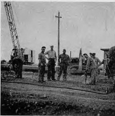
Line ran, reservoir to Pearl Harbor
