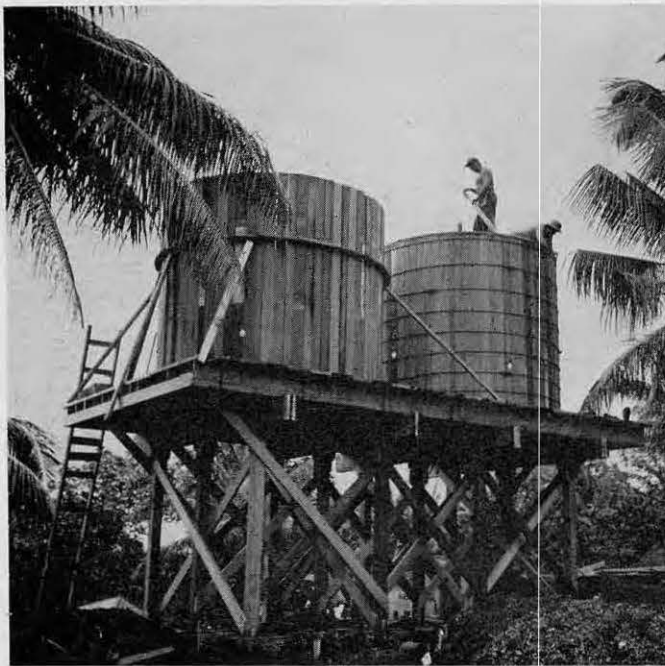
Dual water tanks erected at N. end of Hq. area
