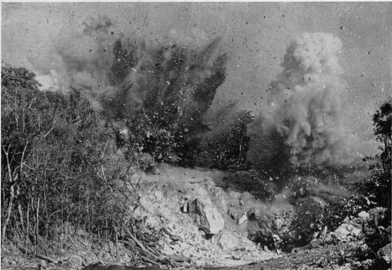
103rd powdermen at rock crusher brought forty per cent glycerine dynamite into use for facing
